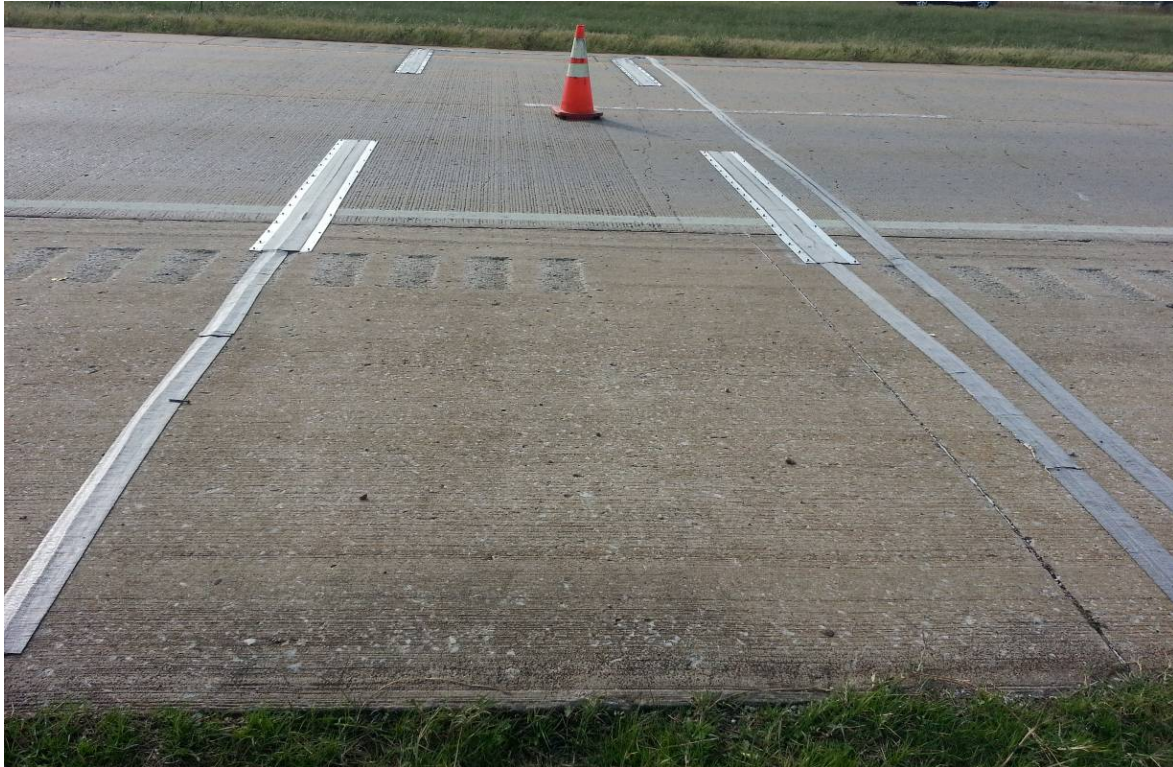
Figure 3.3 Two-lane portable WIM system deployment, near WIM16.
