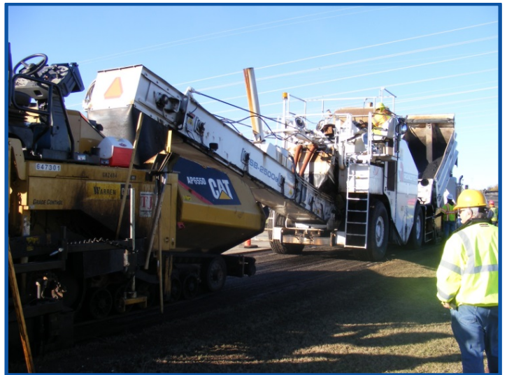
Figure 9. A material transfer device used to construct six overlays in one day
