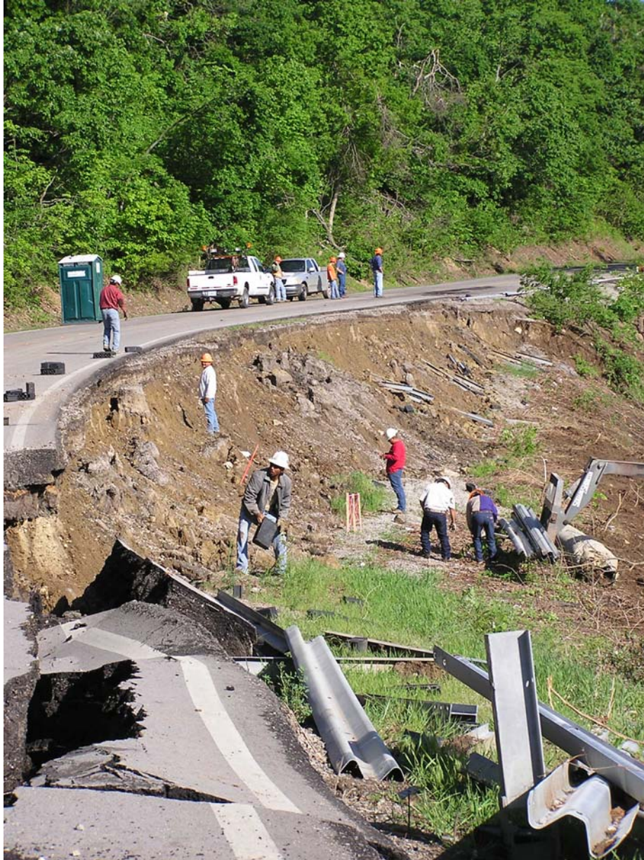
An emergency project to rebuild SH-20 at Keetonville Hill in Rogers County following a slide due to heavy rainfall is being honored with the regional America's Transportation Award. The overall project was scheduled to take 110 calendar days, but crews achieved substantial completion and opened the highway to traffic within 38 days.
